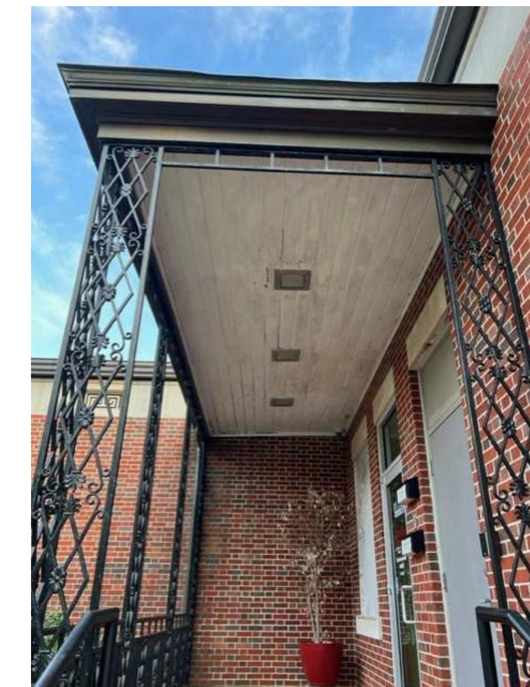
(E) DISPOSE OF WOOD SOFFIT, TRIM, AND LIGHT FIXTURES. PREPARE AREA TO RECEIVE NEW CEILING SYSTEM. COORDINATE WITH THE OWNER TEMPORARILY DISCONNECT SECURITY CAMARA AND REINSTALLATION AFTER COMPLETION OF WORK.
