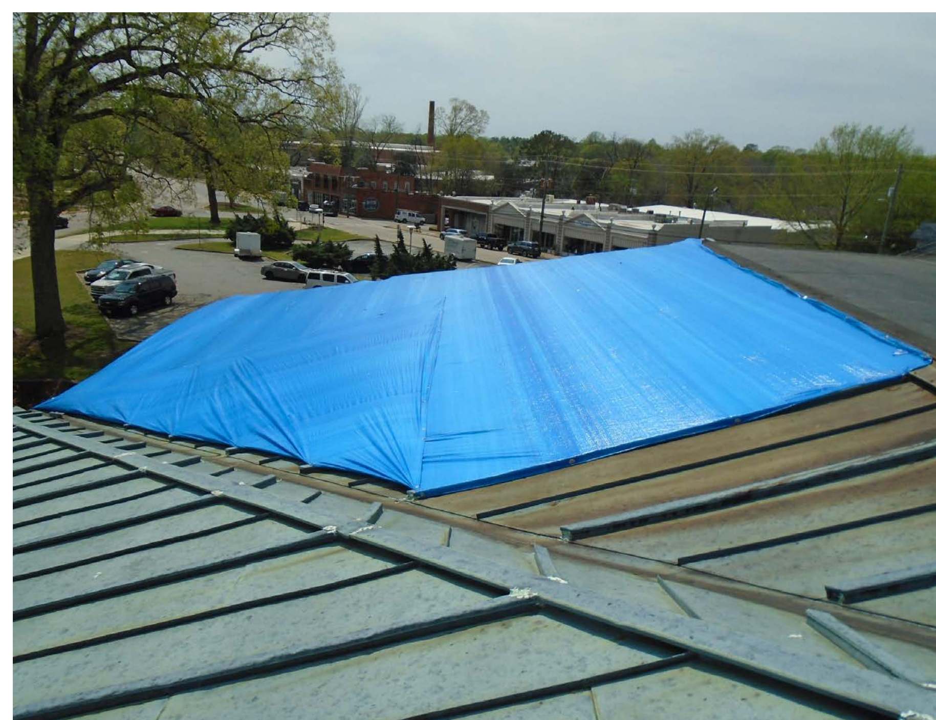
(G) DISPOSE OF TARP. REPLACE ANY DAMAGED TECTUM DECK - MATCH ADJACENT SURFACES. PREPARE AREA TO RECEIVE NEW ROOF SYSTEM.
