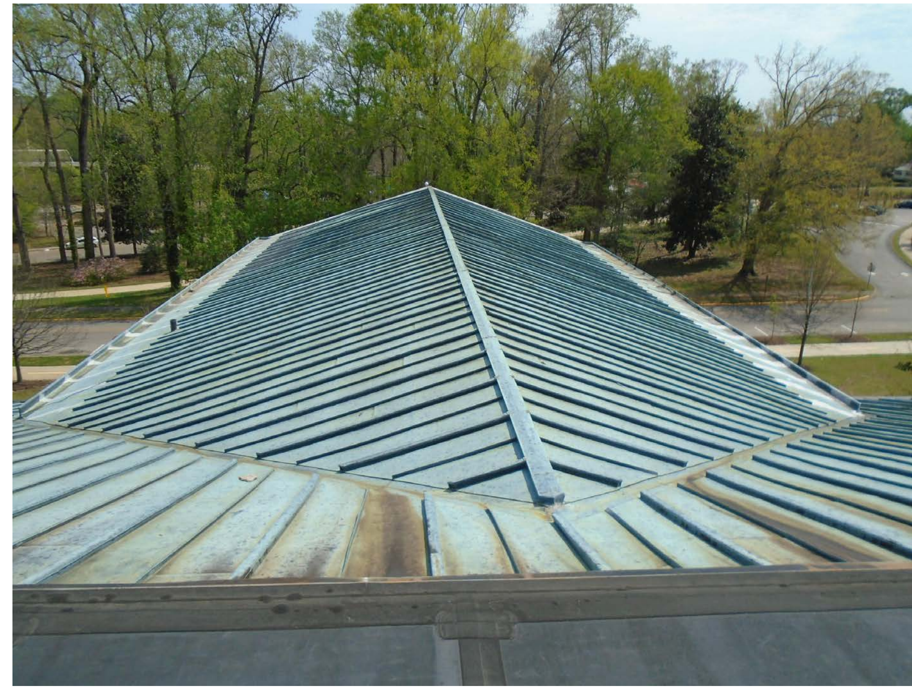
(A) REMOVE AND TURN OVER TO THE OWNER EXISTING COPPER ROOF SYSTEM AND ALL RELATED ITEMS DOWN TO TECTUM DECK.
