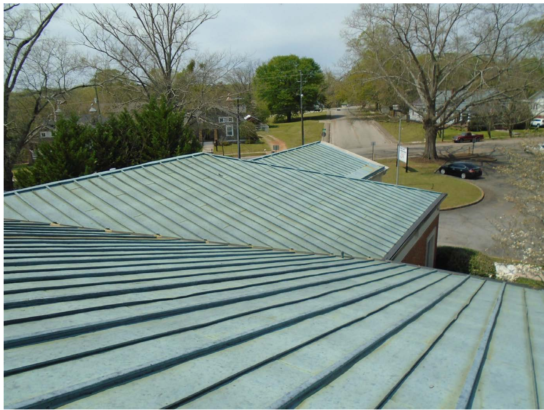
(A) REMOVE AND TURN OVER TO THE OWNER EXISTING COPPER ROOF SYSTEM AND ALL RELATED ITEMS DOWN TO TECTUM DECK.
