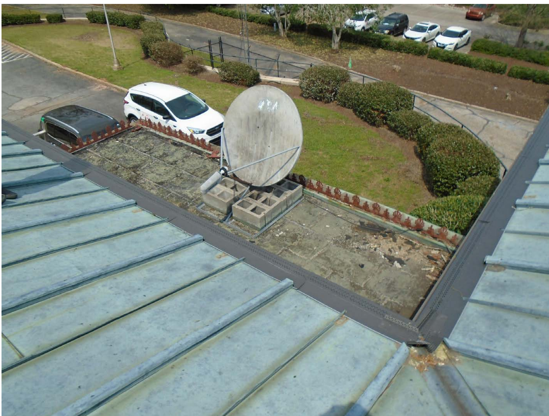
(C) DISPOSE OF CONCRETE BLOCKS, ANTENNA, ROOF SYSTEM, AND ALL RELATED ITEMS. PREPARE AREA TO RECEIVE NEW ROOF SYSTEM.
