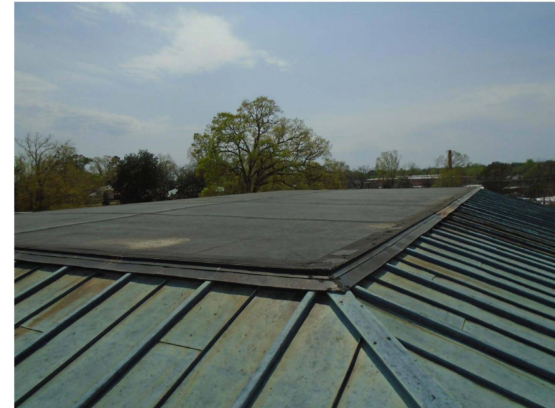
(B) REMOVE AND DISPOSE OF EXISTING MODIFIED BITUMEN ROOF SYSTEM AND ASSOCIATED ITEMS.
